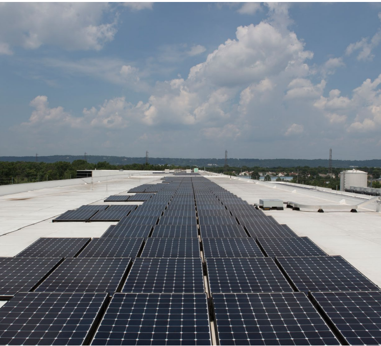
QTS Piscataway Solar Panels
